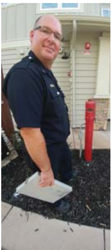
ConFire Capt. Steve Aubert prepares to inspect the post indicator valve. Photos Nick Marnell
